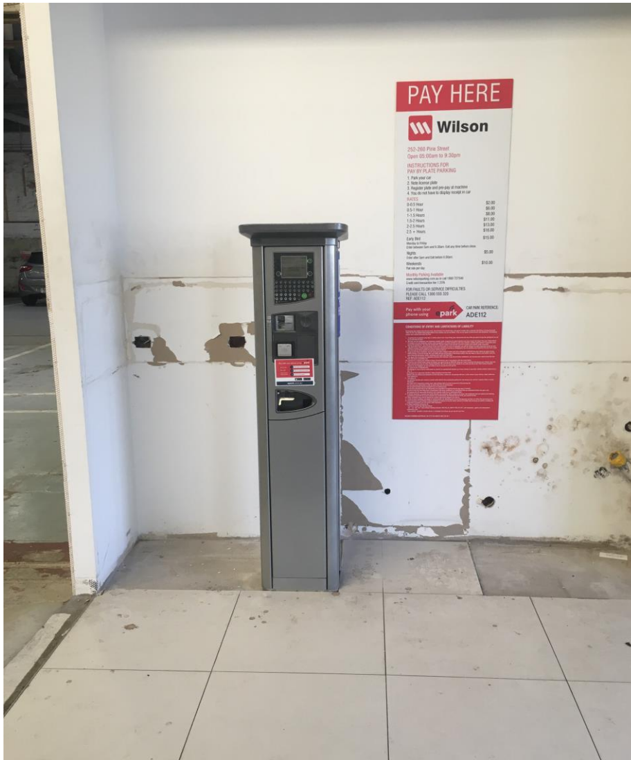
Photo 5 – Existing ticket machine at entrance
